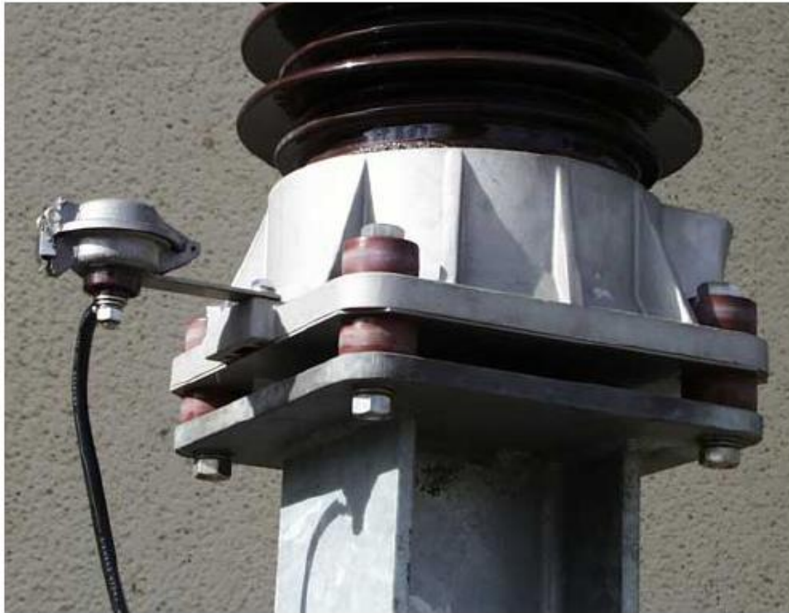
Fig. 13: Bottom flange with insulating feet and monitoring spark gap
