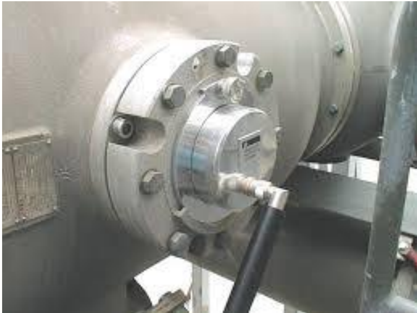
An external window coupler on a 500 kV GIS
