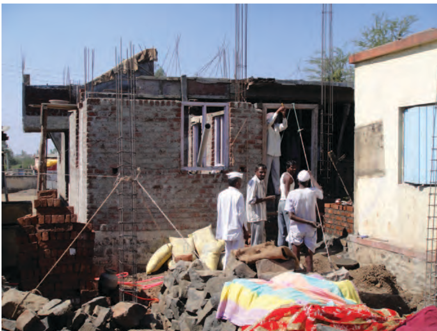
Figure 14. The new constructions in brick and reinforced cement concrete are of very poor quality.
