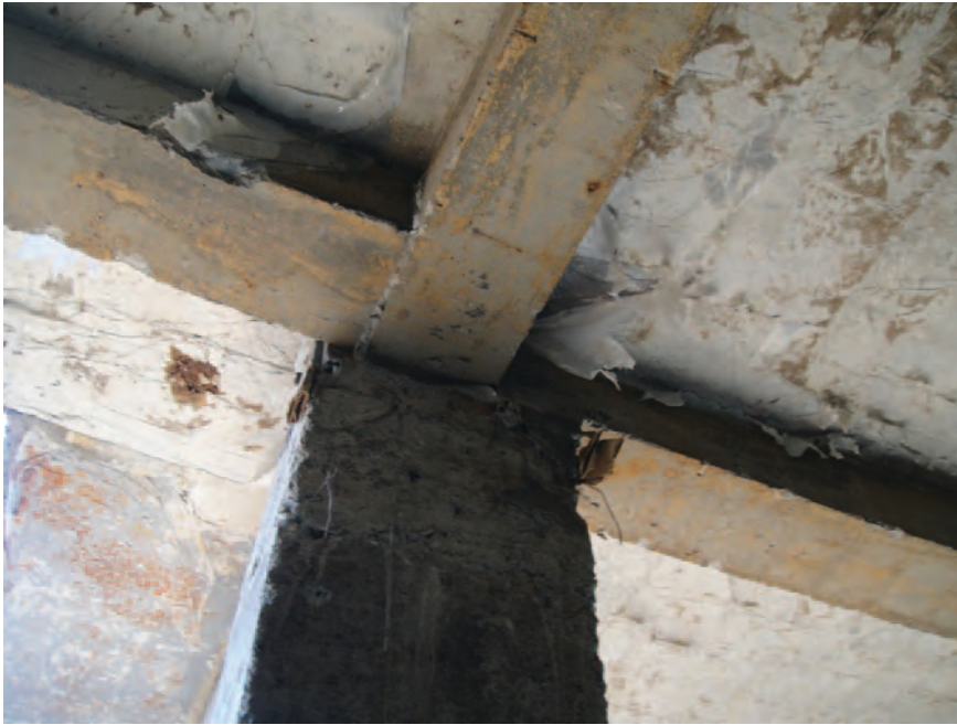
Figure 13. Reinforced concrete columns used for new constructions are of incorrect cross section and do not have adequate reinforcement.
