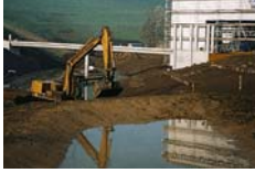
Infiltration swale under construction. Water started to accumulate here even in the building phase.
