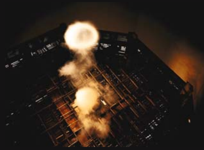
A circular eddy starts to rise from the depths of the cooling tower.
