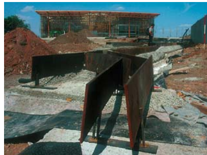
The water fissure under construction, showing the steel structure of the foundations. The Academy is in the background, with the largest solar roof in Europe.
