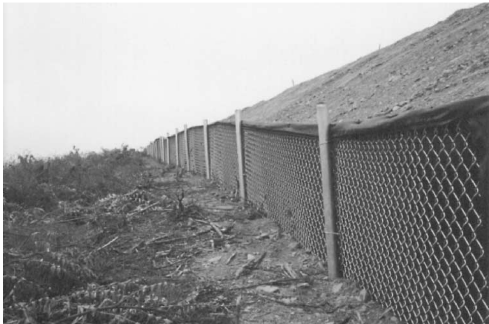
Figure 3.28 Photograph of reinforced filter fabric fence.
