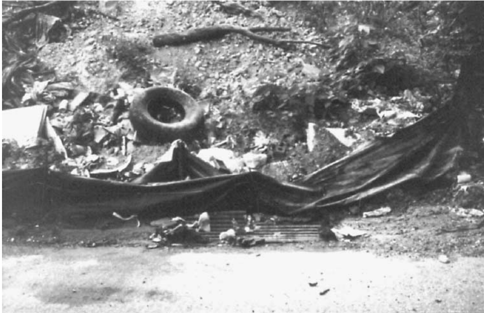
Figure 3.34 Photograph of failed filter fabric fence because of poor maintenance.
