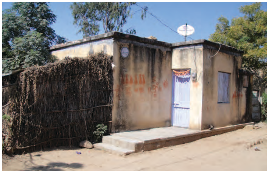
Figure 7. The local people have made additions to the relocated houses using locally-available materials, such as thatch.
