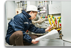
The separation of data and electrical power cabling must comply with safety codes.
