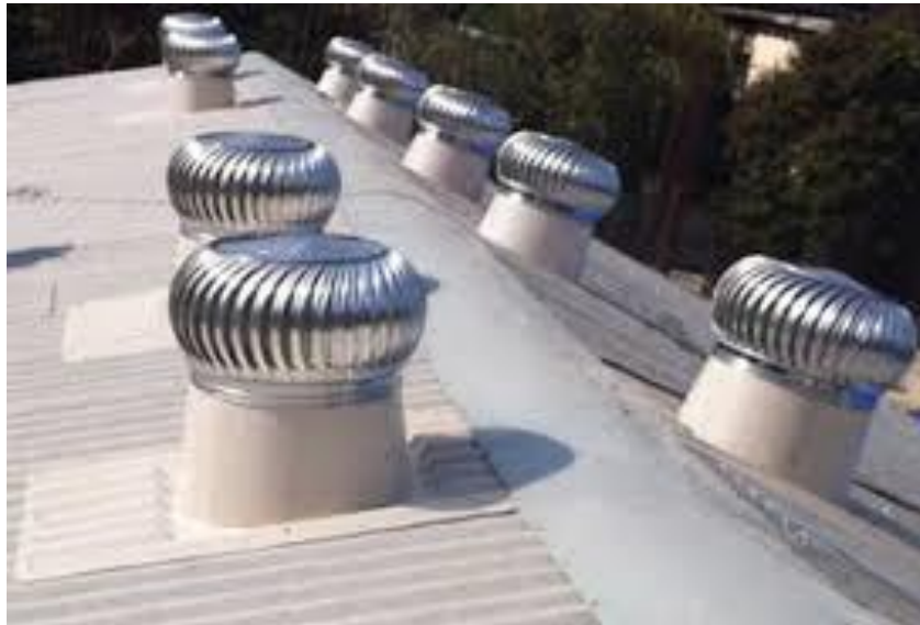
Figure 1: Ventilator Installed at an angle
