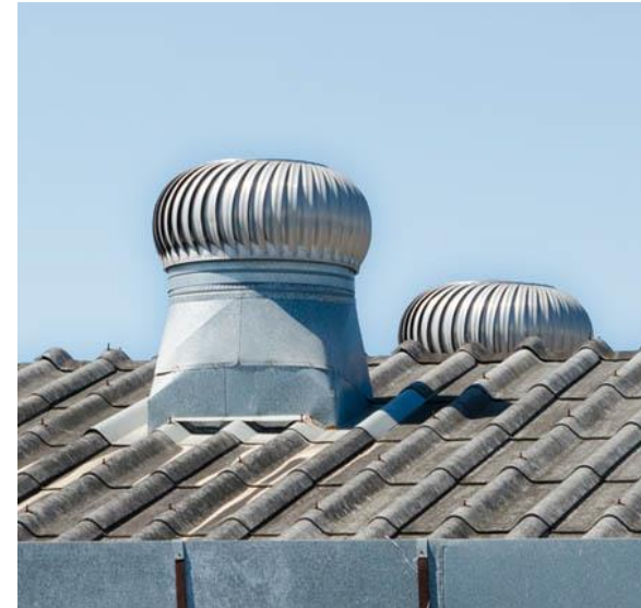
Figure 2: Ventilator Installed at perpendicular to ground
