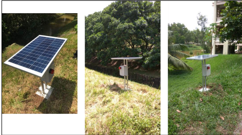
Figure 7.59: Completed installations of the AWAM system for slope monitoring on site
