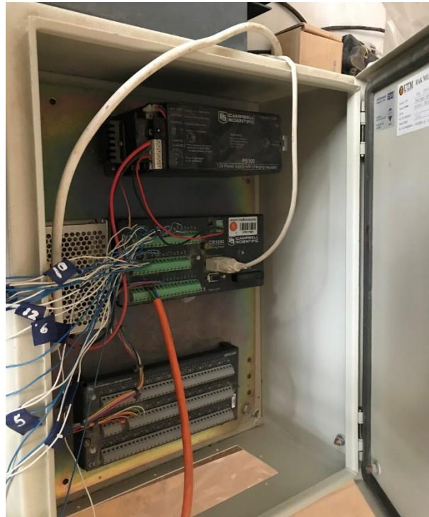
Figure 3.18: The data logger by Campbell Scientific model CR800 used by tensiometers data logging with protruding labelled wires connected to all the tensiometers used in the study
