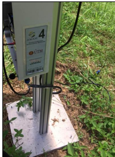
Figure 7.12: Steel base plate supporting the base of the power station
