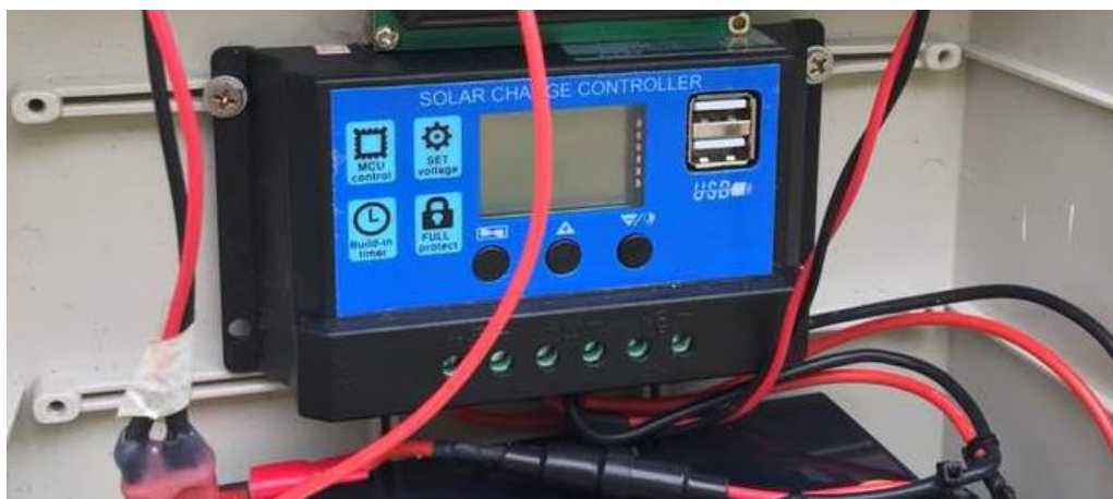
Figure 7.13: Solar charge controller of the power supply
