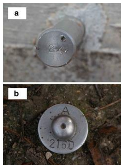
Figure 2.6: Levelling network base point made of stainless steel situated in stable structures (Fastellini et al., 2011)
