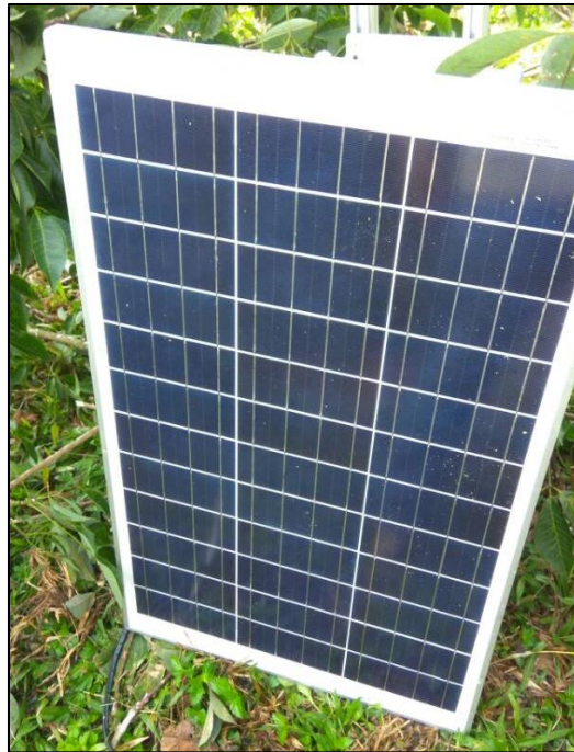
Figure 7.14: Solar panel installed on top of the power station on the AWAM device
