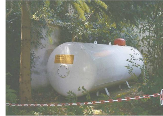
Figure: 08-01-UN Cylindrical pressure vessels, such as this gas tank, have semi-spherical end caps rather than flat ones in order to reduce the stress in the tank.
