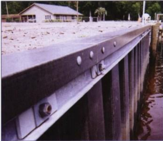
Complete composite sheetpile installation, including SuperLoc™ sheetpile and composite top cap. (Picture courtesy of Creative Pultrusions.)
