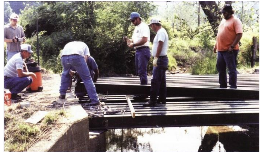
Steel flange beams were replaced by pultruded FRP beams, reinforced with carbon fibres in the flanges to increase stiffness to over 6 million psi, in this bridge upgrade in Blacksburg, Virginia.
