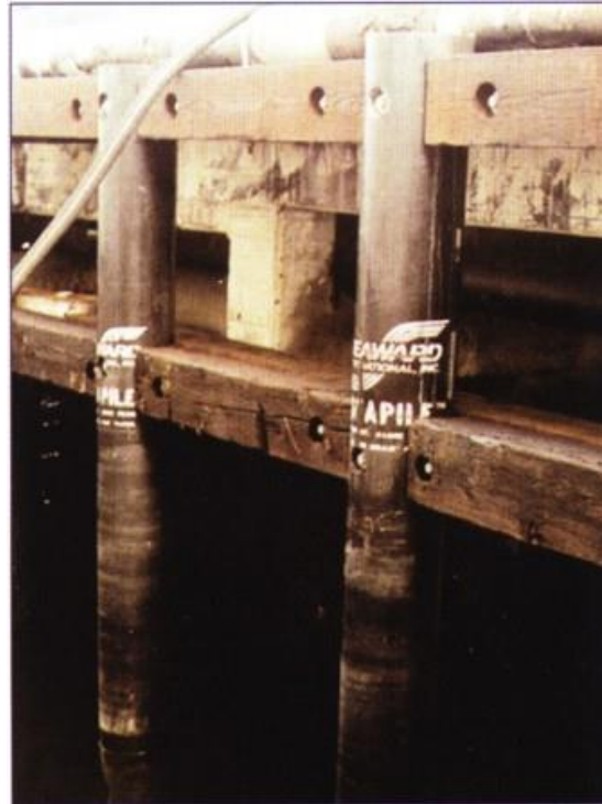
Navy pier structure made using pultrusion. (Picture courtesy of Owens Corning: www.owenscorning.com .)
