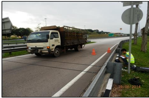
Figure 2 Installation of Automatic Traffic Counter at the entry point of Machap Rest and Service Area
