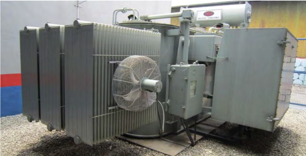
30 MVA, 33/11 kV power transformer in distribution substation
