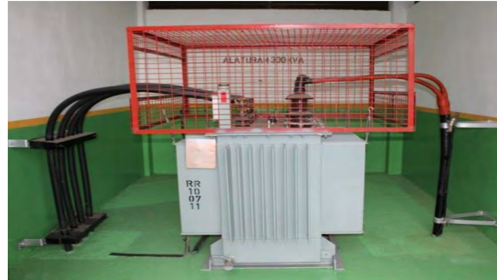
300 kVA, 11/0.433 kV distribution transformer in electrical substation
