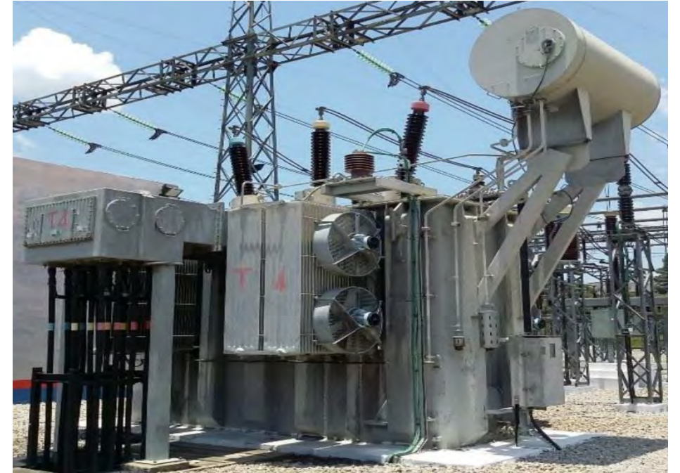
45 MVA, 132/33 kV power transformer in intake substation
