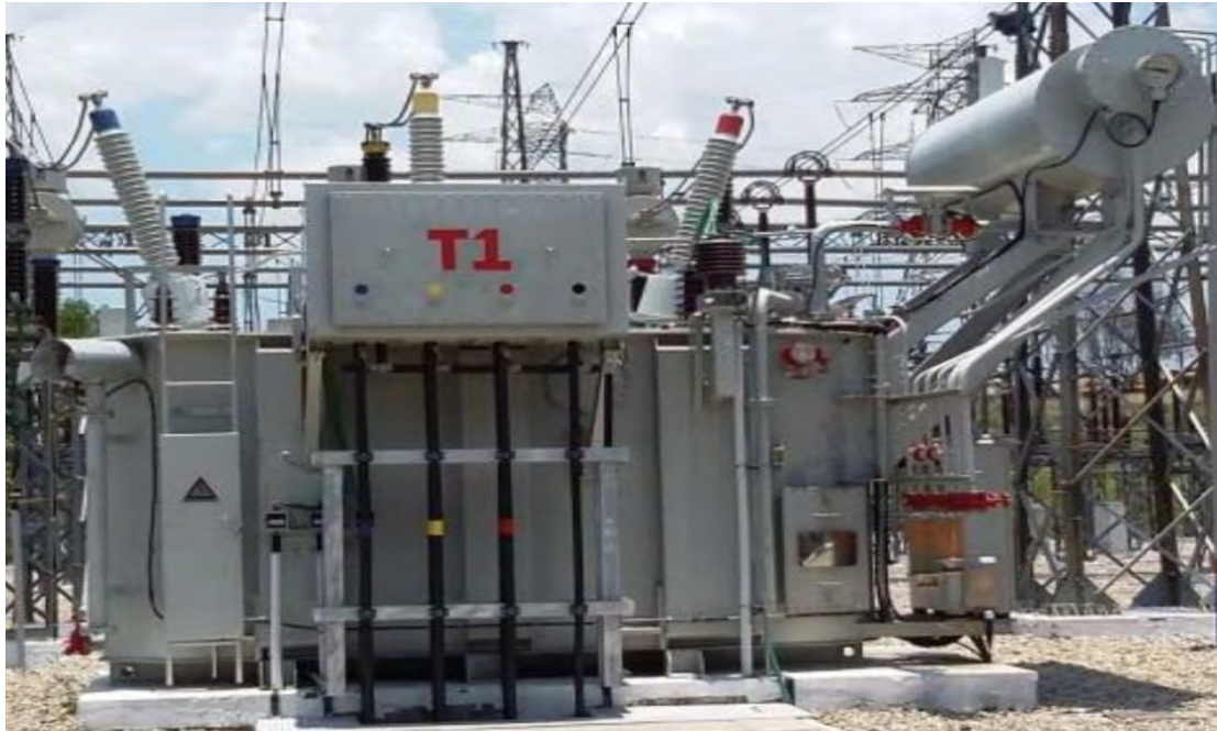
30 MVA, 132/11 kV power transformer in intake substation
